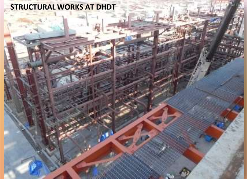
HEATER WORKS FOR DHDT
